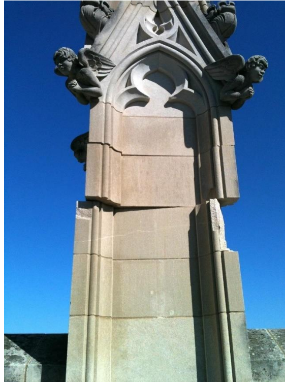
Figure 26: Earthquake Damage to Washington National Cathedral in Washington, D.C. After the 2011 Earthquake 78
